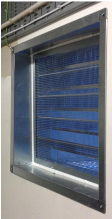
Fig. 7: Mounted backdraught damper in wall
