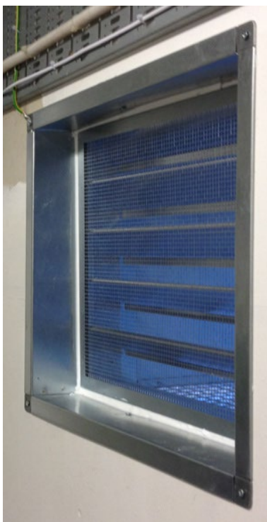
Fig. 7: Mounted backdraught damper in wall
